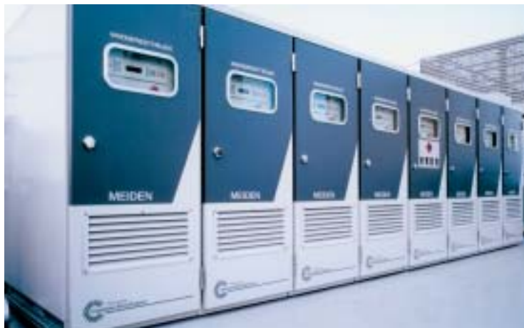
Example of a 200+ kilowatt array of Capstone MicroTurbine driven Sumitomo-Meiden combined heat and power systems atop a hospital in Oita, Japan.
