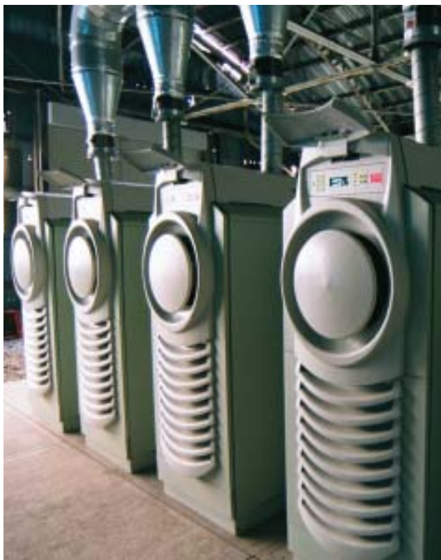
An array of microturbines at a closed coal mine in Japan turns methane into power while exhausting the CO 2 back into the mine.
