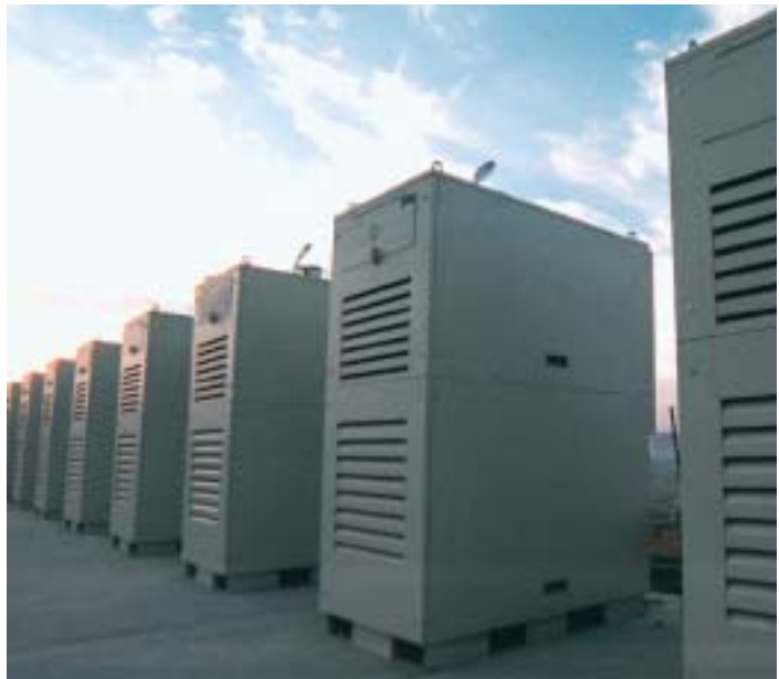
Landfill gas fuels several microturbine arrays in California and elsewhere.
