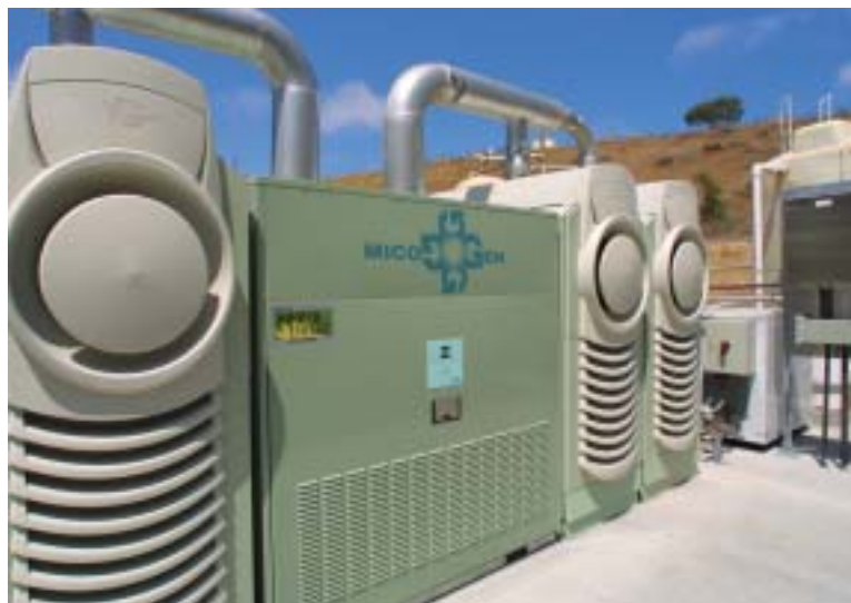
Microturbines at sewage plants create power from biogas while exhaust heat maintains temperature of the sewage digester vats.
